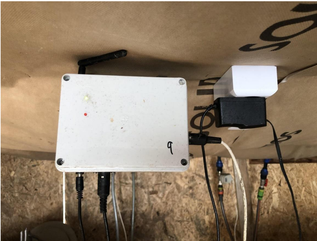
Smart client installed to ceiling
