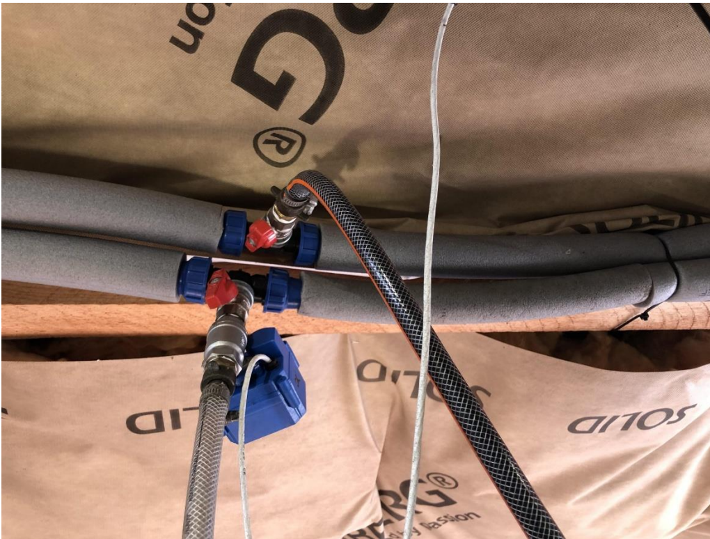
Servo valve installed into cooling system
